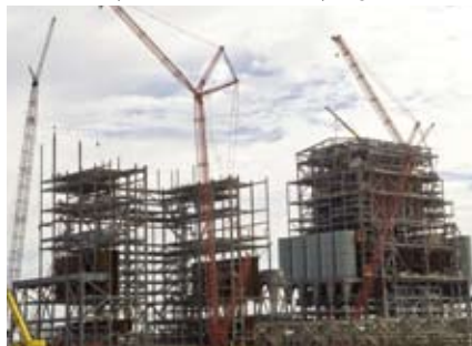
The Luminant Oak Grove Power Plant, a clean coal technology power plant for which Fluor is performing EPC and commissioning. Oak Grove, TX.
