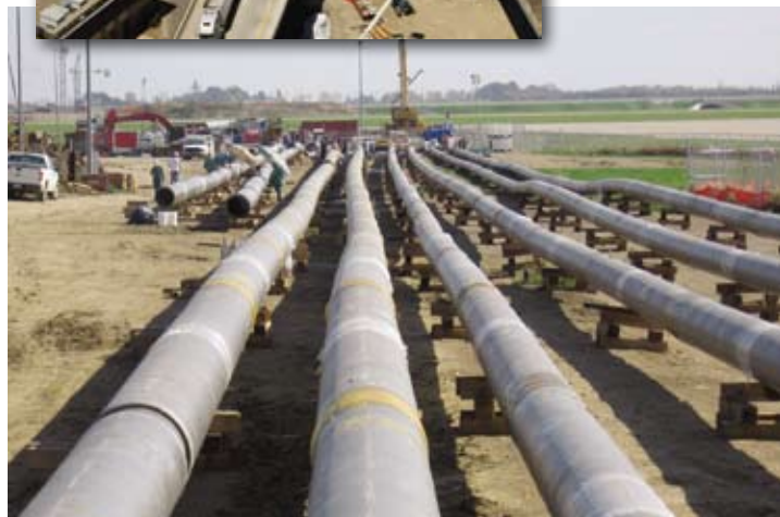
AGC 2008 Aon Build America Award Winner, Bowen Engineering Corporation. This photo showcases the Central Energy Plant Indianapolis Maintenance Center Utility Connector, Indianapolis, IN.
