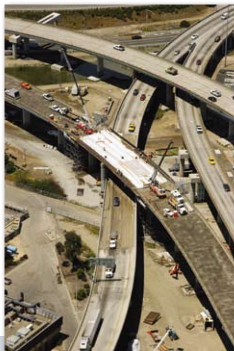
AGC 2008 Aon Build America Grand Award Winner, the I-580/880 Emergency Repair by C.C. Myers, Inc., in Oakland and Emeryville, CA.
