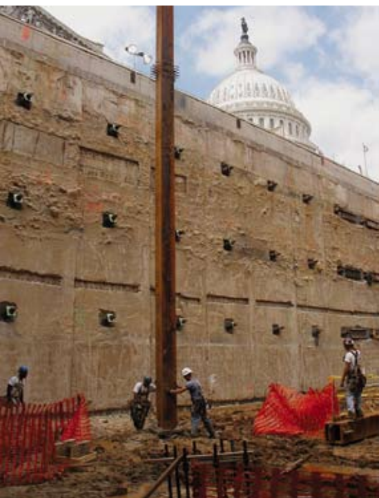
In all, 494 tie-backs were installed through the perimeter wall at the Capitol Visitor Center, ensuring its stability against the tremendous pressure exerted on it by the weight of the Capitol and surrounding earth.
